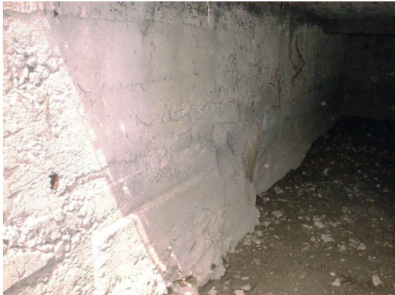
Figure 4. Lack of insulation, visible numerous irregularities, honey-combings in concrete and fragment of left shuttering
