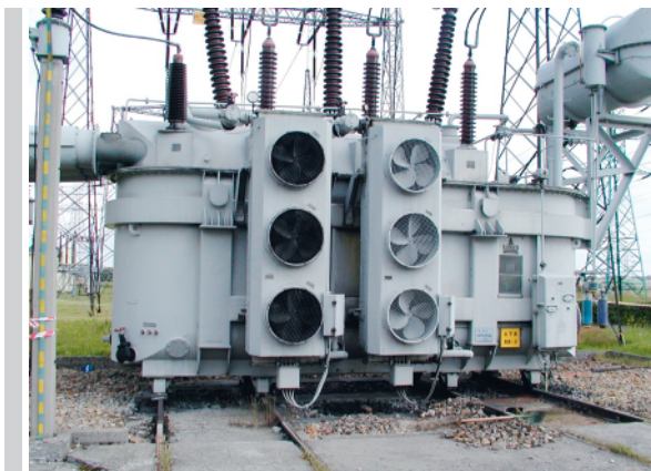
Figure 2. 220/110 kV transformer on a work station
