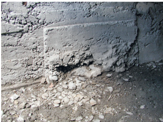
Figure 5. Lack of insulation, visible defects of concreting
