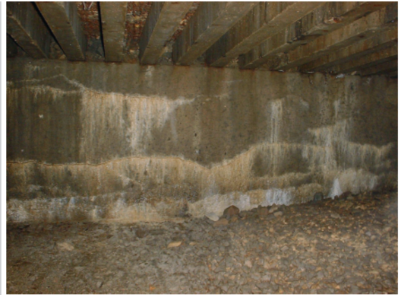
Figure 6. Heavy horizontal cracking of an oil tank wall, traces of ground water leakage
