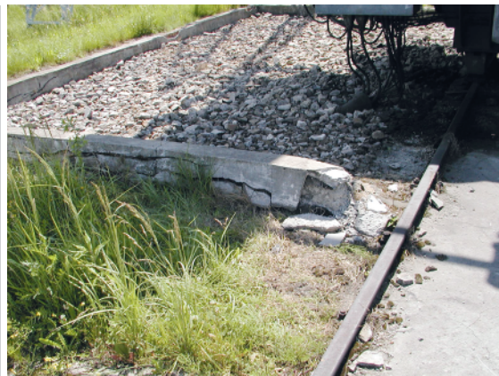
Figure 9. Substantial damage to upper section of an oil tank wall, lack of the drivable section filling
