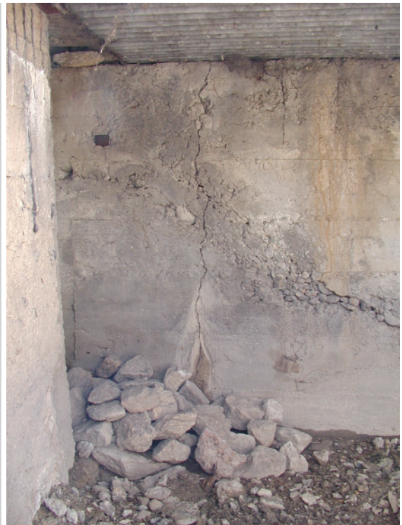
Figure 7. Heavy vertical cracking of an oil tank wall, concrete sorting out, traces of leakages
