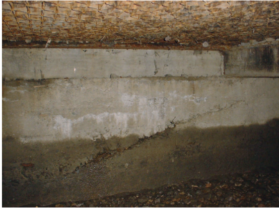
Figure 3. Lack of a wall insulation, visible defective contact between concrete layers and dampness
