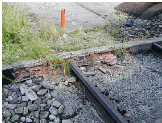
Figure 10. Damaged brick filling of transit section of the wall
