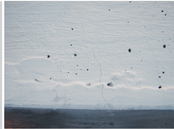
Figure 9. Cracked beam II-2
