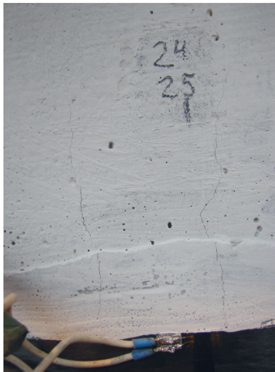
Figure 8. Cracked beam II-1
