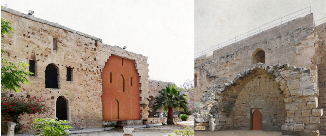
Figure 3. Closing the gap in the eastern rooms of Kyrenia Castle with Corten and new access to the Eastern fighting gallery and Venetian filling [16]
