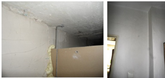
Figure 7. Cracking of the walls and ceilings inside the building
