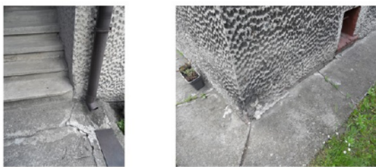
Figure 8. Cracking of the entrance stairs and the splash apron around the building
