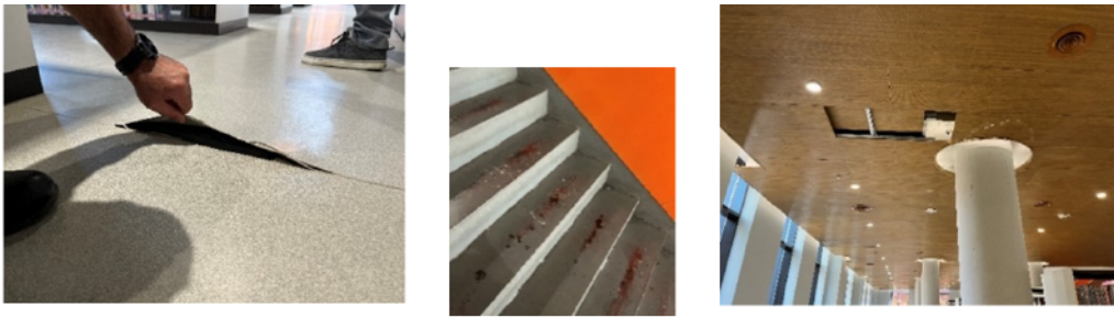
Figure 12. Deformed floor covering material, deformed step, and deformed ceiling covering material (Photos by the authors)
