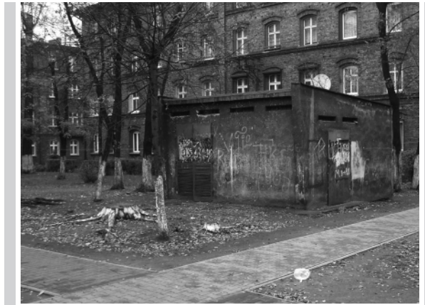
Figure 13. Katowice Załęże – graffiti on the transformers station building in the vicinity of the playground. Photo taken by the author
