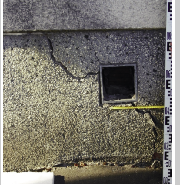
Figure 4. 2 cm cracks in a foundation wall as a result of a shrinkage ( \Delta s=5 cm) of the expansive clay, settlement of a concrete band ( \Delta s=10 cm)
