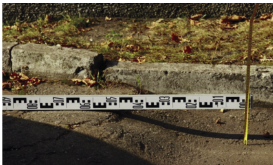
Figure 7. Raising of a manhole as a result of expansive base swelling ( \Delta s = 22 cm)
