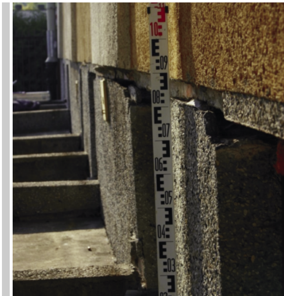
Figure 3. An example of a building failure as a result of cyclical swelling-shrinkage. Maximum lowering of the foundation wall ( \Delta s=10 cm)
