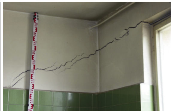
Figure 6. An example of wall damage, an outer view
