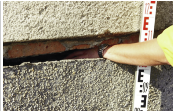
Figure 5. An example of damage to a foundation wall, an outer view
