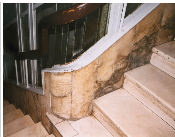
Figure 12. Warsaw, tenement house at Marszałkowska 18 ( L. Korngold, 1935-1936 ) – stairs (alabaster), lift (glass and metal)
