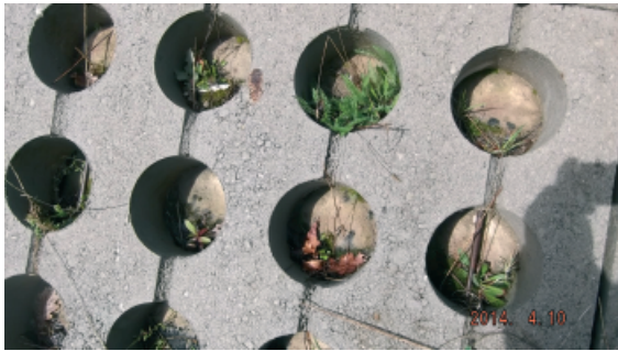
Figure 6. Openings in concrete plates with geotextile on the bottom side (private collection)
