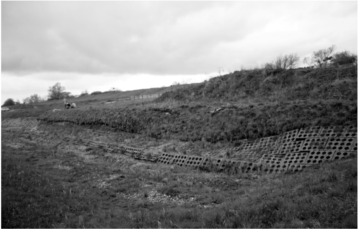
Figure 2. View of the slope after the failure (private collection)
