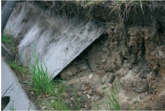
Figure 5. Hollow space below the geotextile caused by moving the soil to the gravel layer located underneath the concrete plates (private collection)
