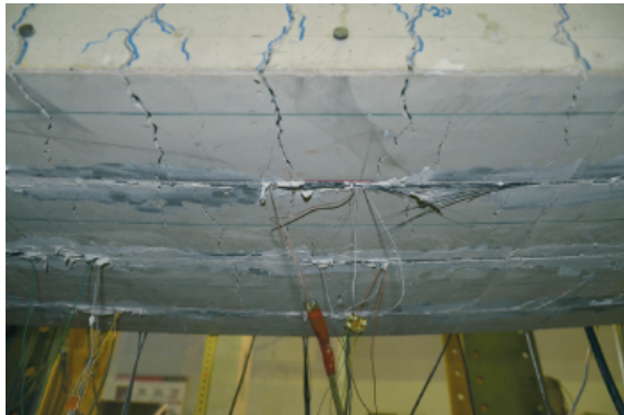
Figure 5. Rupture of the passive CFRP strip
