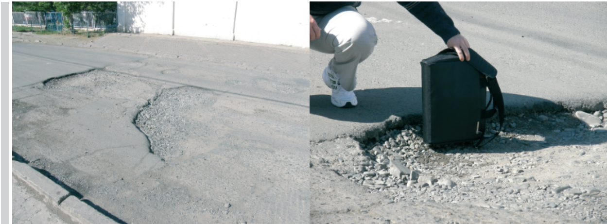
Figure 1. Bad road conditions with potholes
