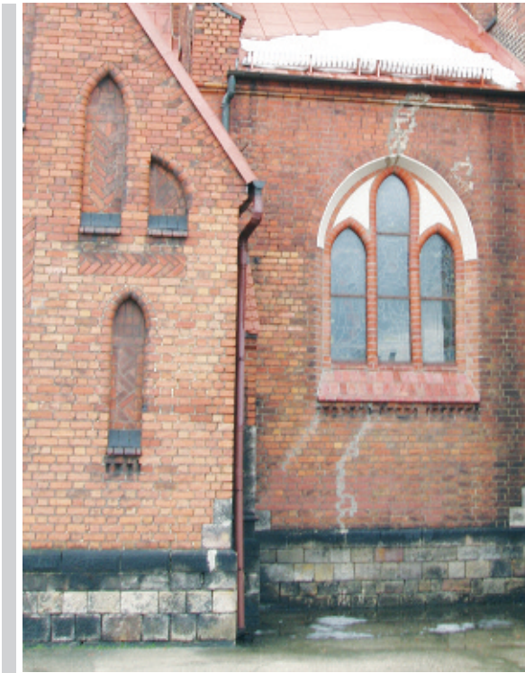
Figure 15. Cracked protective plate and church's exterior wall
