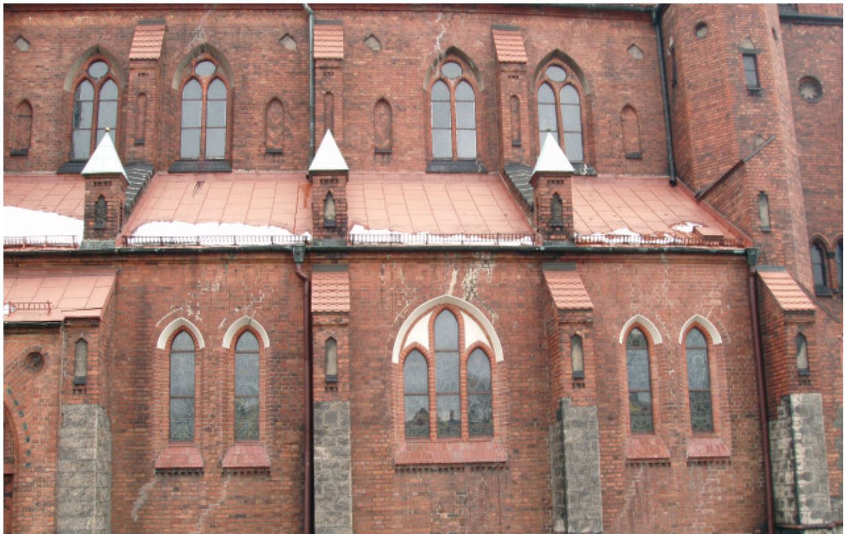
Figure 16. Damage to church's exterior walls
