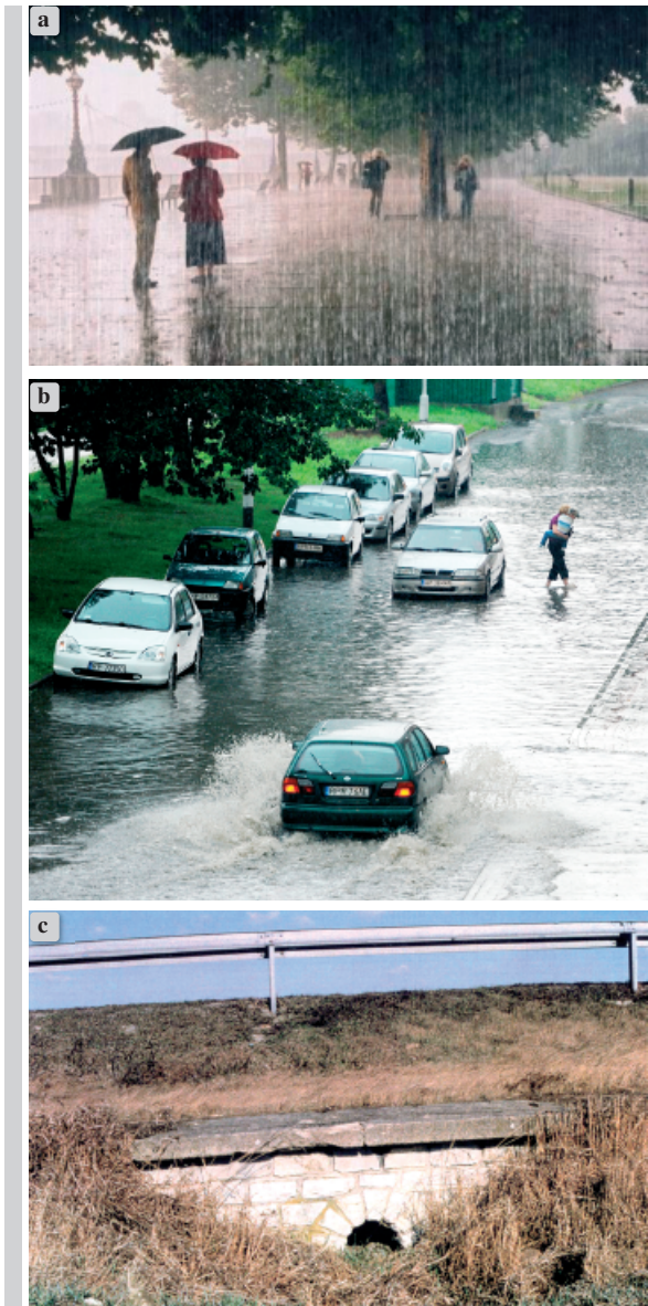
Figure 1. a) High intensity rainfall, b) The Flood after rainfalls, c) Example of faulty culverts
