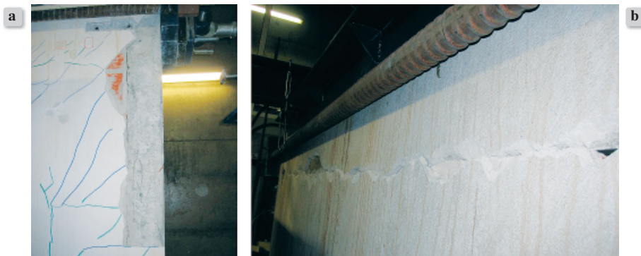
Figure 19. In-plane apparent state of damage: a) lateral interface; b) upper interface
