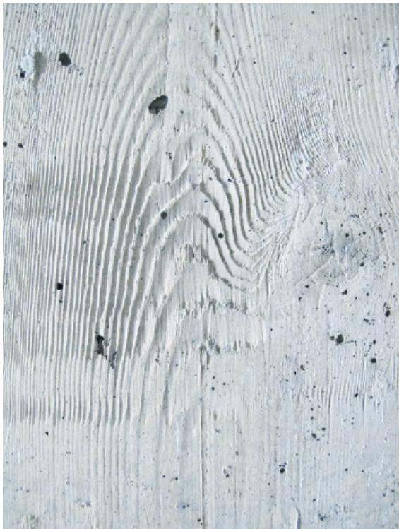
Figure 12. METU Department of Architecture Building – concrete texture with the imprint of the wooden formwork [photo: H. Zelef]
