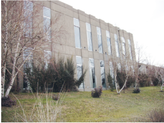
Figure 7. METU Department of Architecture Building – fragment of the north elevation [photo: W. Niebrzydowski]
