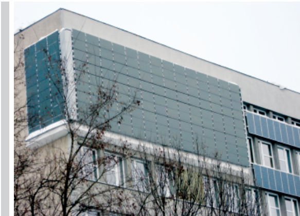
Figure 11. PV modules installed on facade – Environmental Engineering Faculty building in Warsaw (photo J. Tymkiewicz)
