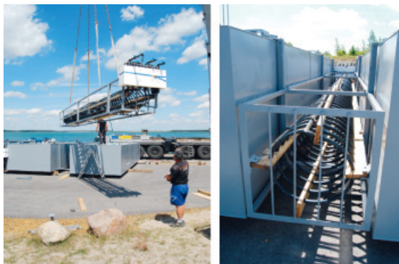
Figure 15. Fitting of heat exchanger in the pontoons for cooling and heating of the floating house according to Fig. 5
