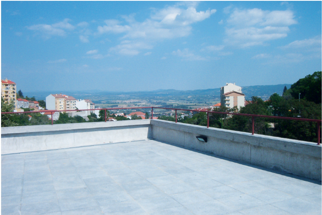
Figure 15. The open space of a terrace created on the roof of the university library. This area gives the possibilities to enjoy the remote view of the Ribeira da Goldra River valley in Covilha. Photo: The author
