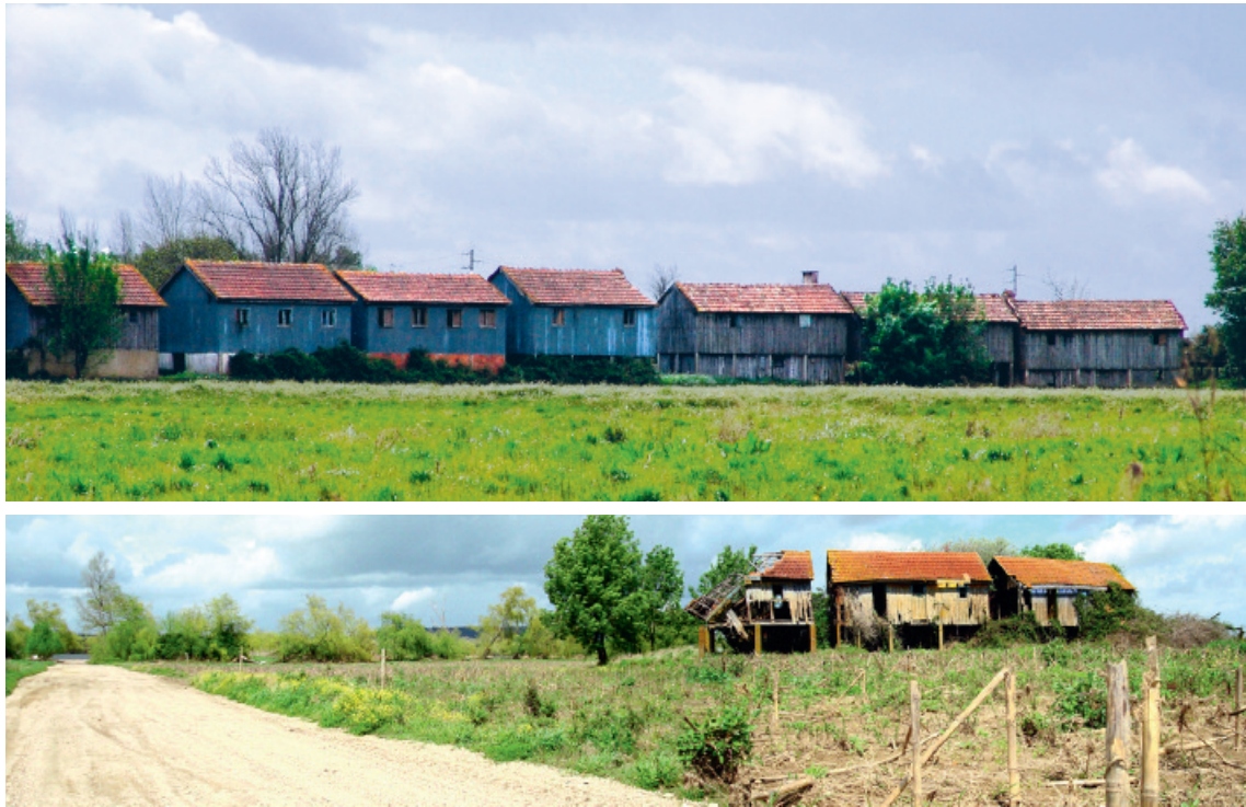
Figure 1. An example of deterioration and abandoning of Portuguese heritage. The case of Patacão, a wooden village near the Tagus River (photos by Filipa Almeida and Filipa Navarro)
