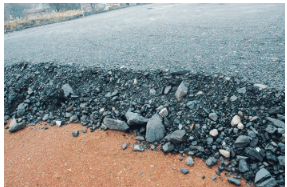
Figure 5. Construction of Bytom ring road. Embankment layer made of unburned spoil laid on a layer of burned spoil (author Krzysztof Chlipalski, Ph.D. Eng.)
