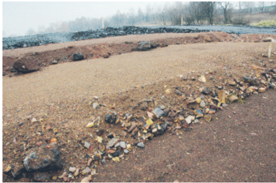
Figure 6. Construction of Bytom ring road. Layers of embankment made of burned and unburned spoil (author Krzysztof Chlipalski, Ph.D. Eng.)
