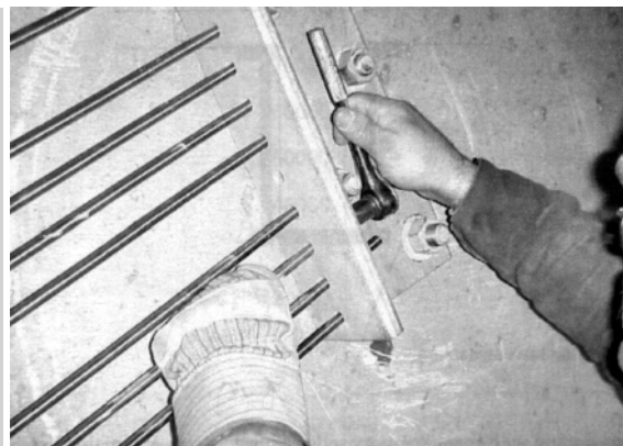
Figure 10. Assembly of SMA rods for external strengthening of a bridge (taken from [14])
