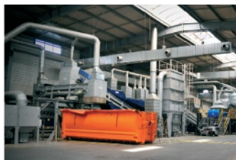
Large-sized waste Plant
